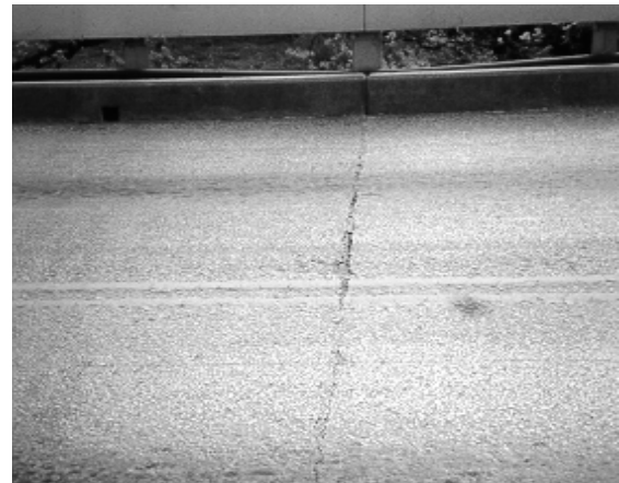
Figure 4.17 Cracked Slab over Floor Beam
